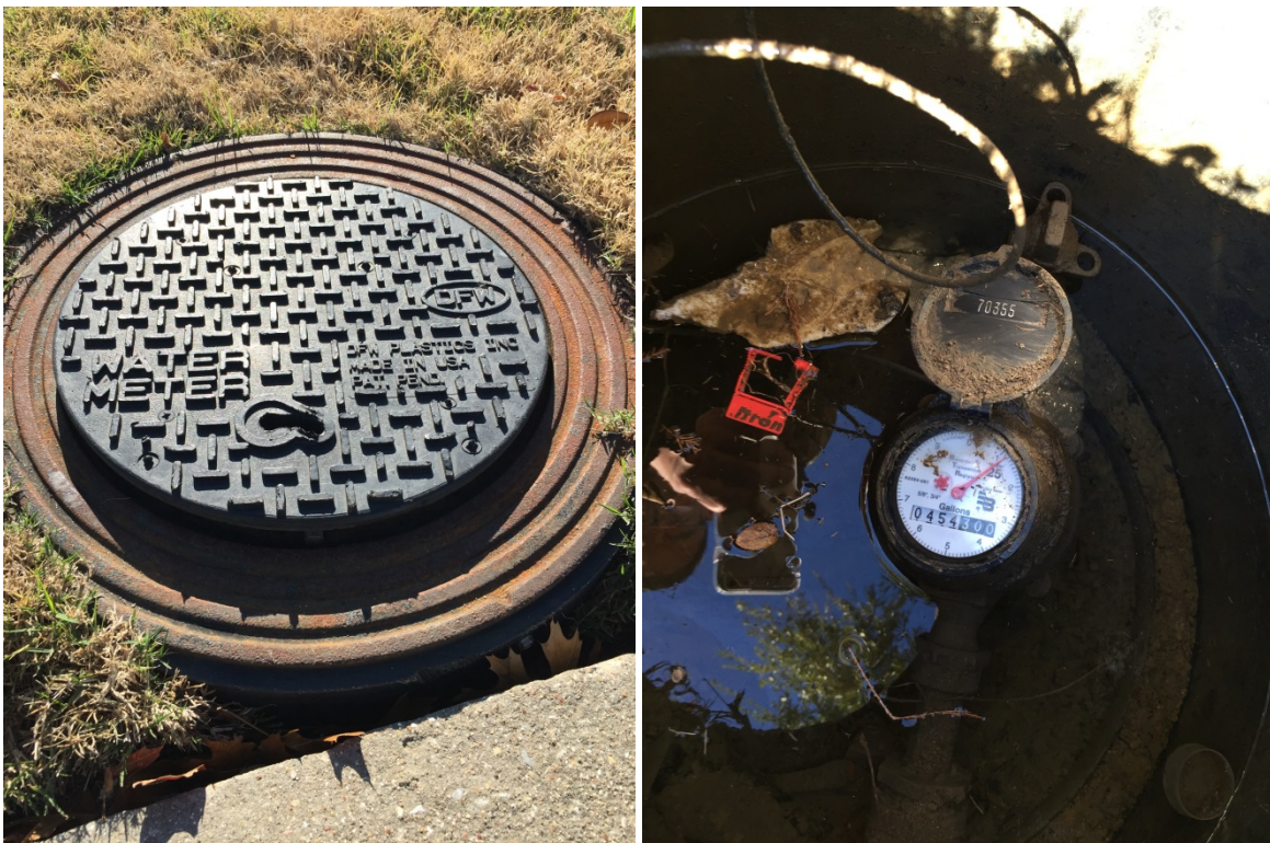
Left is a picture of an unlocked water meter box which houses the water meter and register. It must be located and unlocked with a meter box key for manual reads. On the Right, an uncovered meter box reveals the register dials which are read and the water usage is manually keyed into an electronic handheld device.
