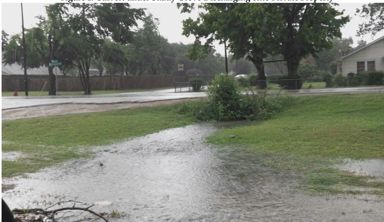
Figure 2: Culvert under Shady Grove Discharging onto Private Property
