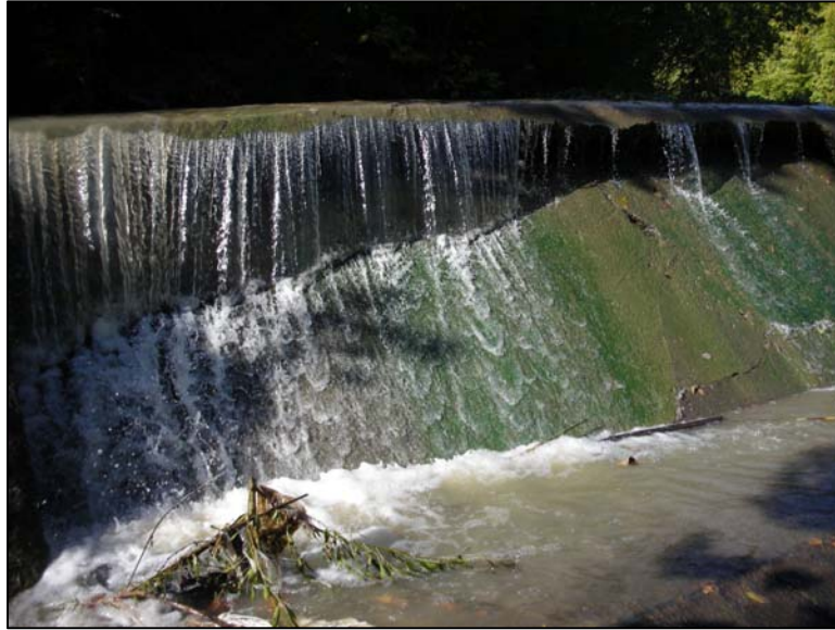
Photograph IX-5: Concrete Failure on Downstream Side of Inline Structure #3
