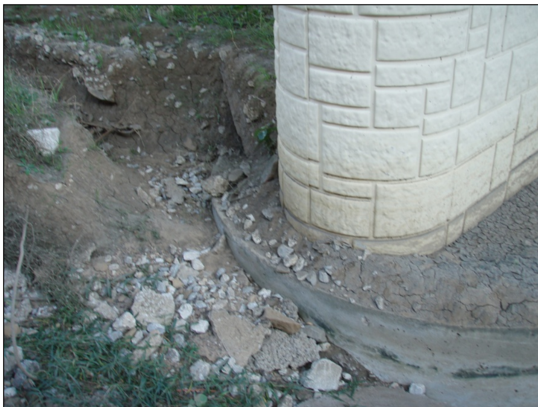
Photograph IX-9: Pier Scour at SH 161 Caused Footing to Become Exposed
