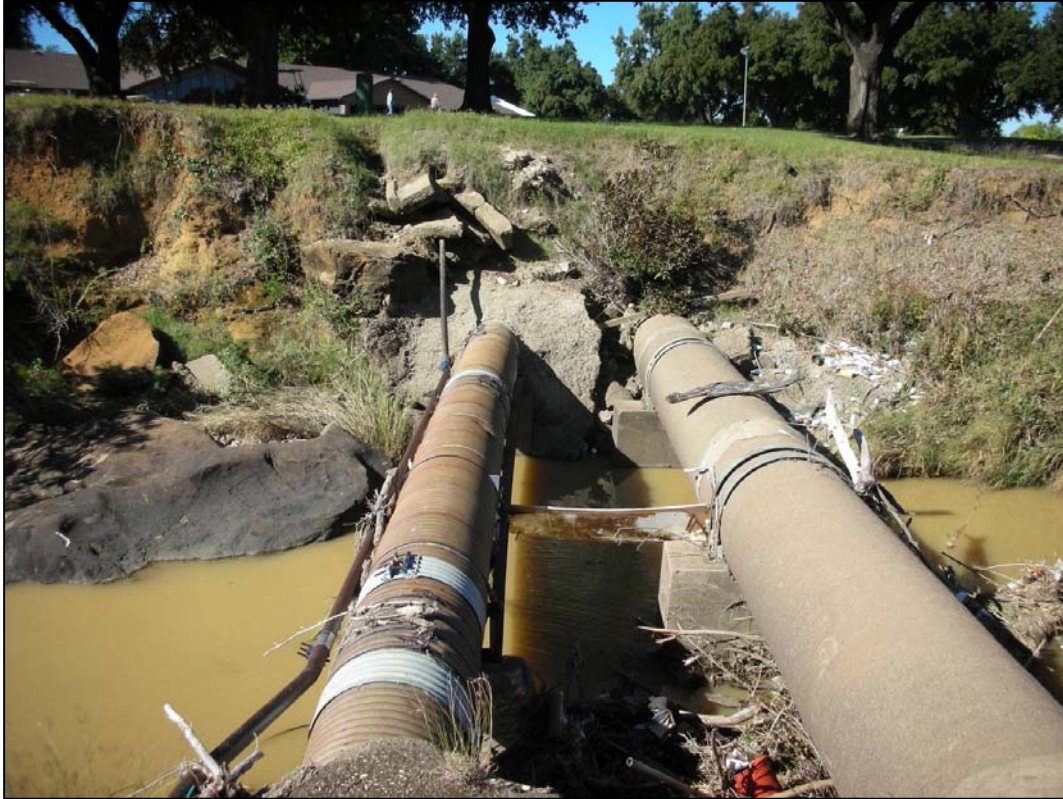
Photograph IX-2: Slope and Concrete Failure at Aerial Crossing #2
