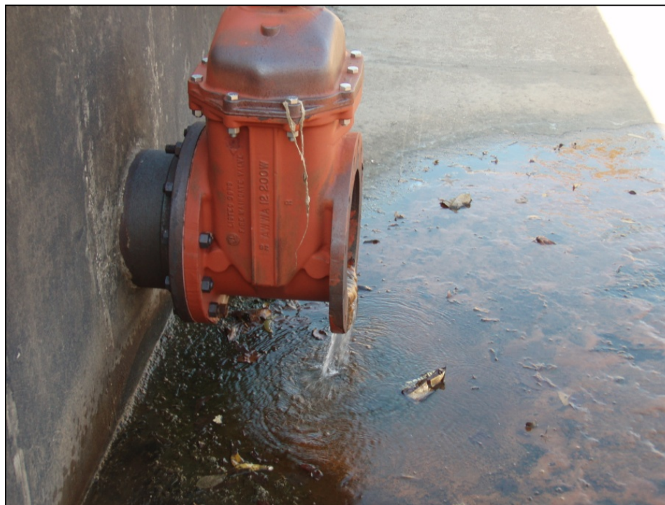
Photograph IX-11: Water control Valve on Downstream Side of Inline Structure #5. Valve is fully opened but is clogged with sediment
