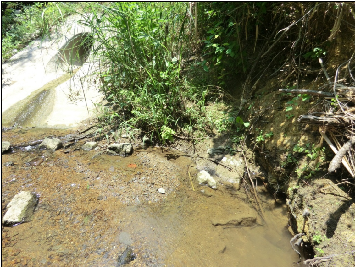
Figure 4.6 Looking upstream at bank erosion near cross section 3491
