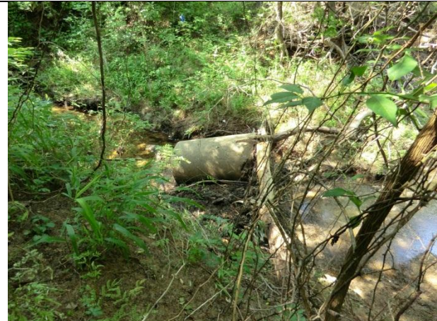
Upstream of 1153 there was a debris jam around a segment of concrete pipe.
