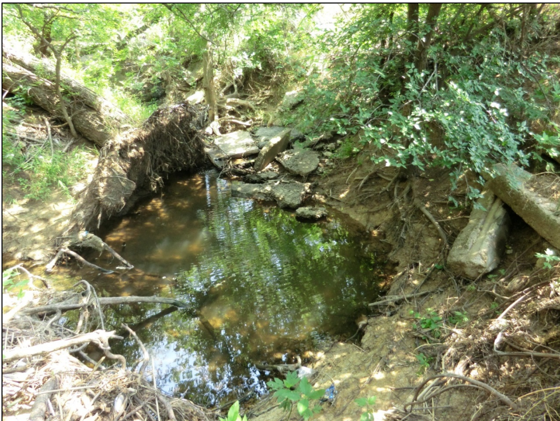
Figure 4.8 Looking upstream at the undercut concrete crossing and severe erosion near cross section 2496
