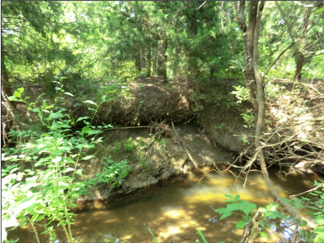
Figure 4.9 Looking downstream at a slump failure on the right bank downstream of the scoured concrete crossing near cross section 2496
