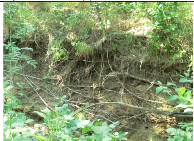
Right bank downstream of 1153 the banks are actively eroding.
