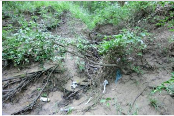
Upstream of 37902 outfall, gully erosion
