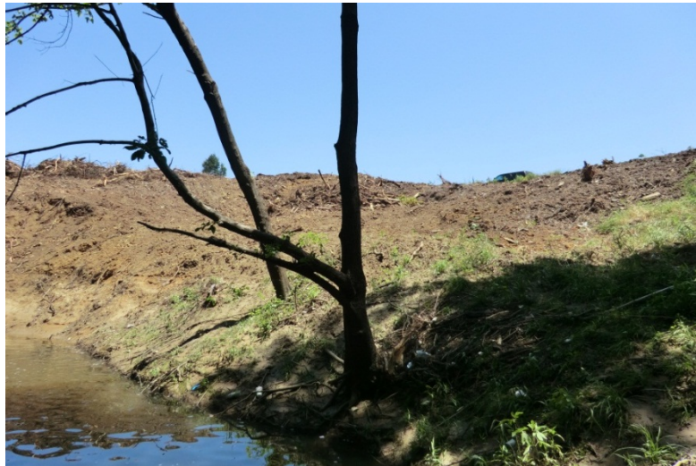
Figure IX-7: Bank Erosion at Cross Section 252+91
