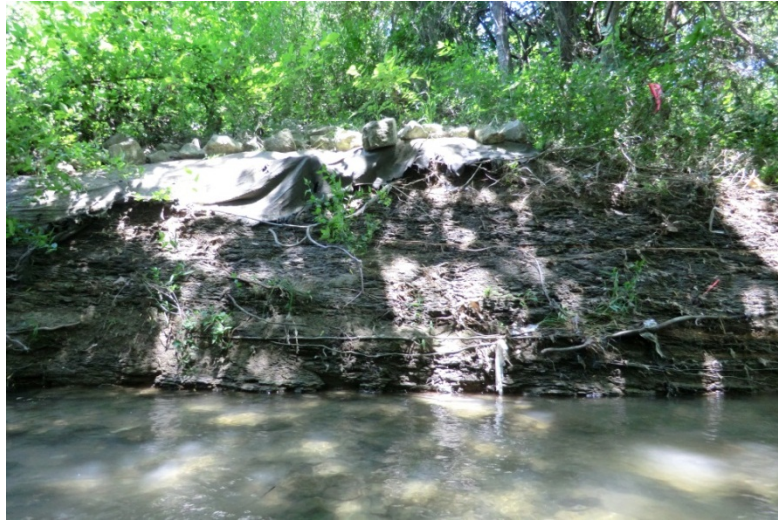
Figure IX-11: Bank Erosion at Cross Section 180+97
