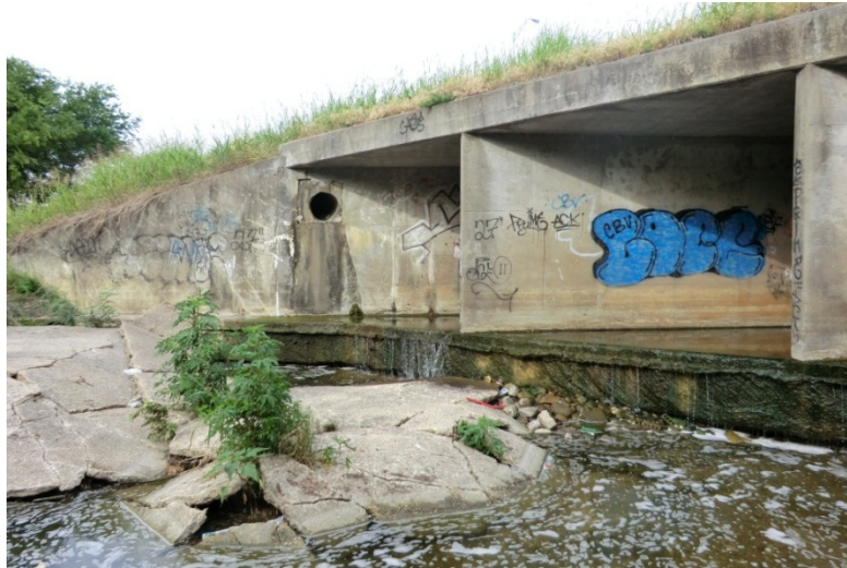
Figure IX-9: Downstream Culvert Damage at SH-360
