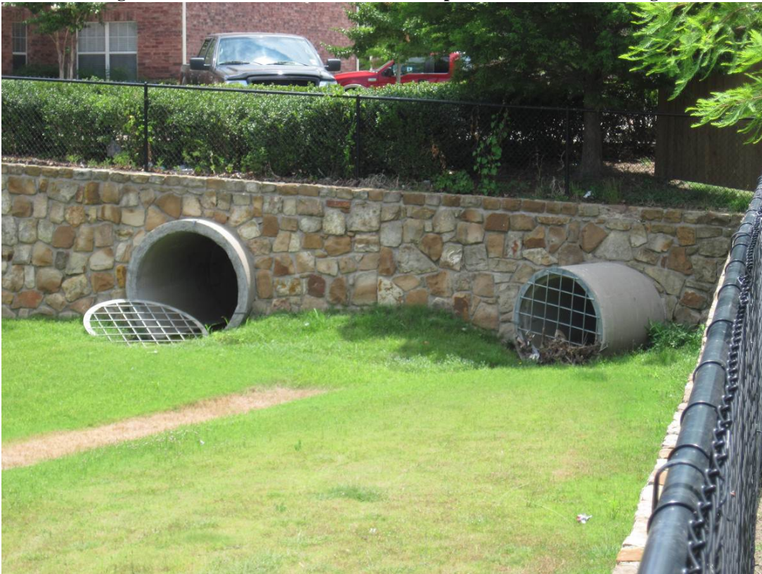
Figure X-13: FC Detention Pond No. 11: Apartments off I-20 Frontage
