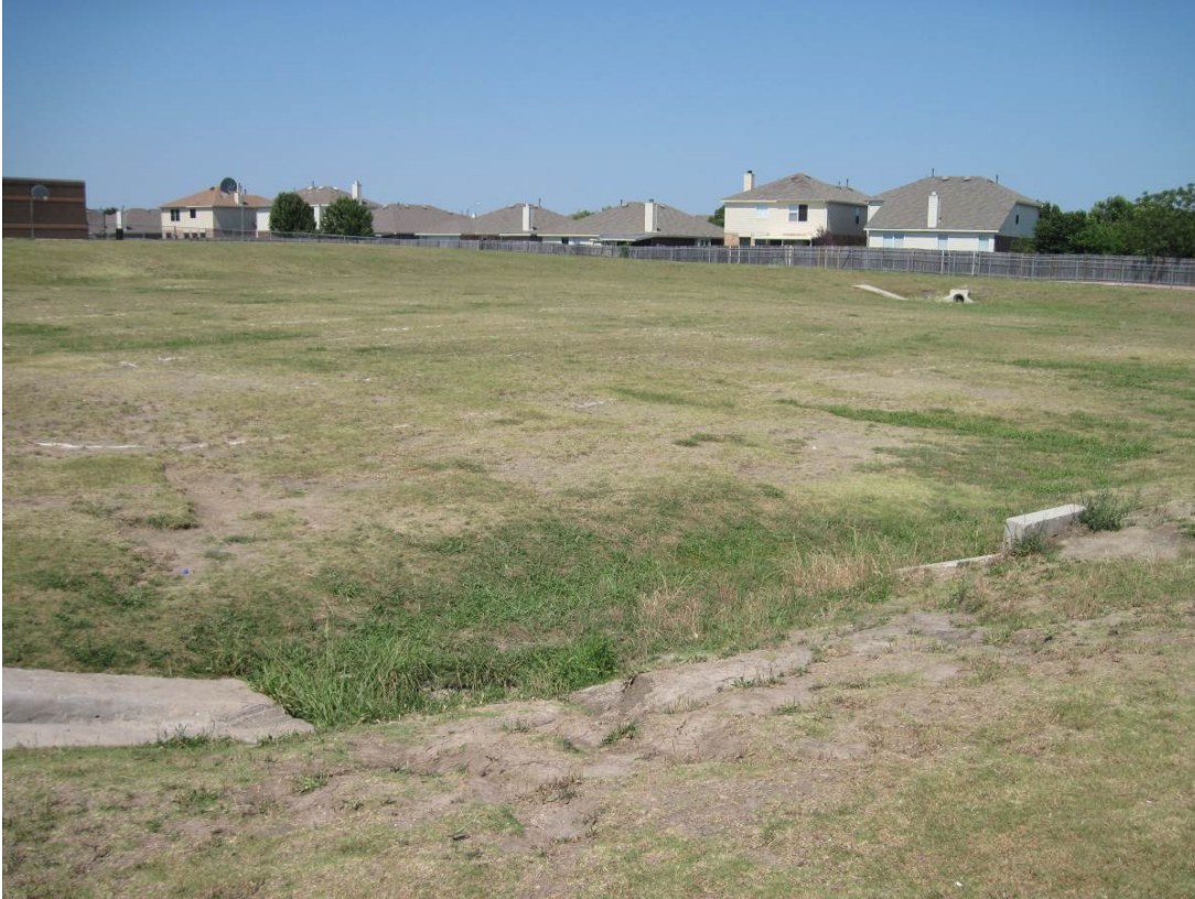
Figure X-4: FC Detention Pond No. 3: Thurgood Marshall Elementary School
