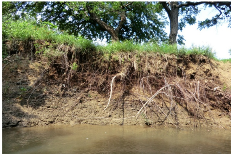
Figure IX-10: Bank Erosion at Cross Section 210+69
