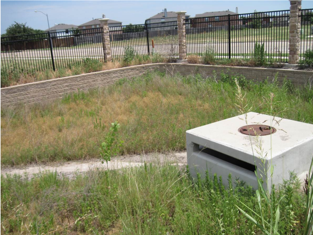
Figure X-15: FC Detention Pond No. 13: Westside of Magna Carta just North of Camp Wisdom
