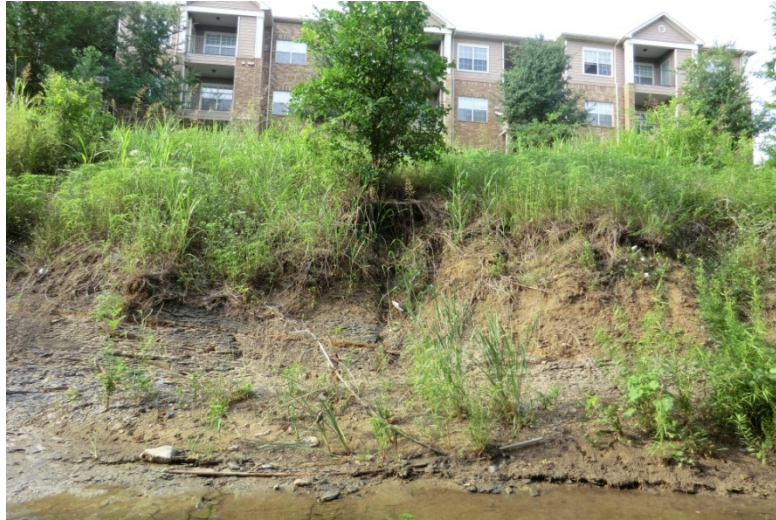
Figure IX-13: Bank Erosion at Cross Section 132+76
