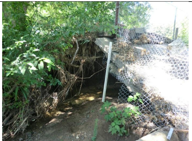
At 2272 there was a concrete low water crossing that was severely undercut.
