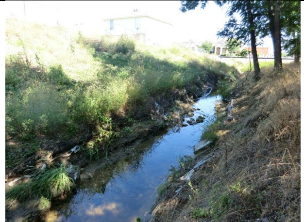
Upstream view from 4526, scour on the banks and the erosion matting was showing.
