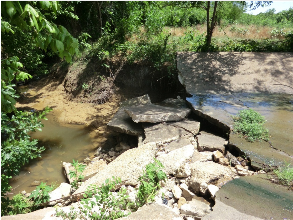
Figure 4.8 Looking downstream at the undercut concrete spillway and severe erosion near cross section 881
