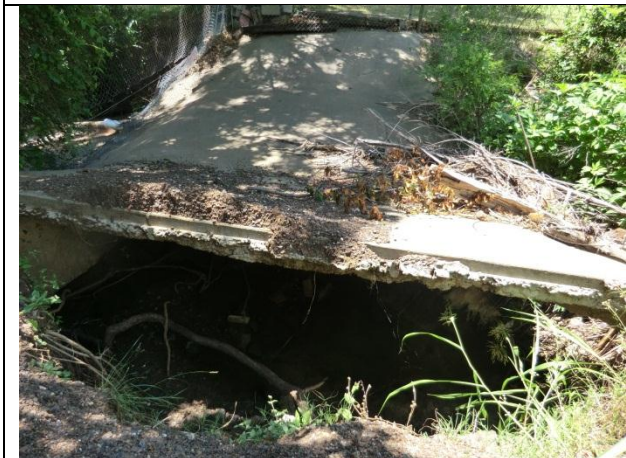
At 2272 there was a concrete low water crossing that was severely undercut.
