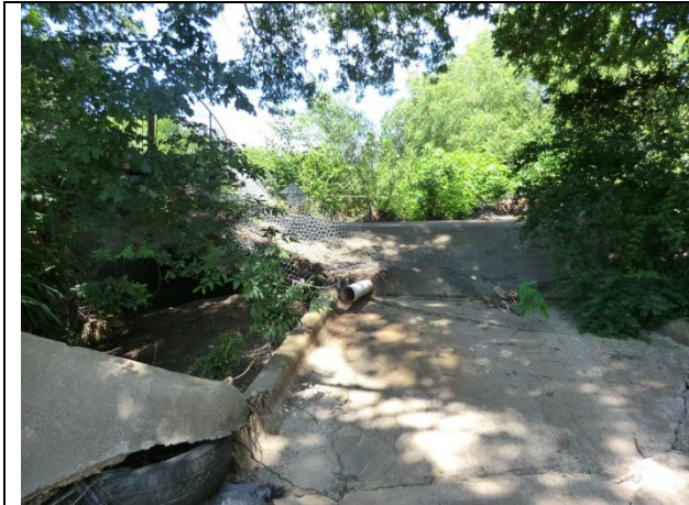
Upstream view from 2228 shows a cracked and undercut low water crossing/drop structure.
