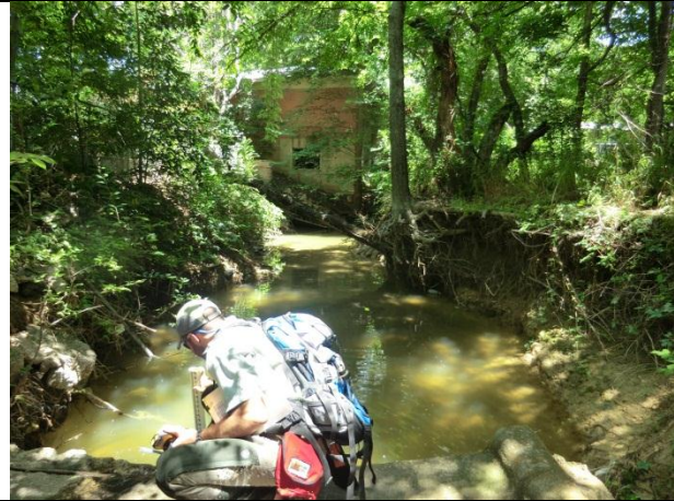
Downstream view from 2062 shows a 4-foot drop from the concrete to the channel bed and severe erosion downstream.
