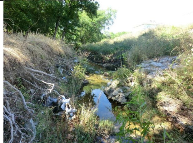
Downstream view towards 4526, bank scour on the left bank from a riprap slope (outfall).
