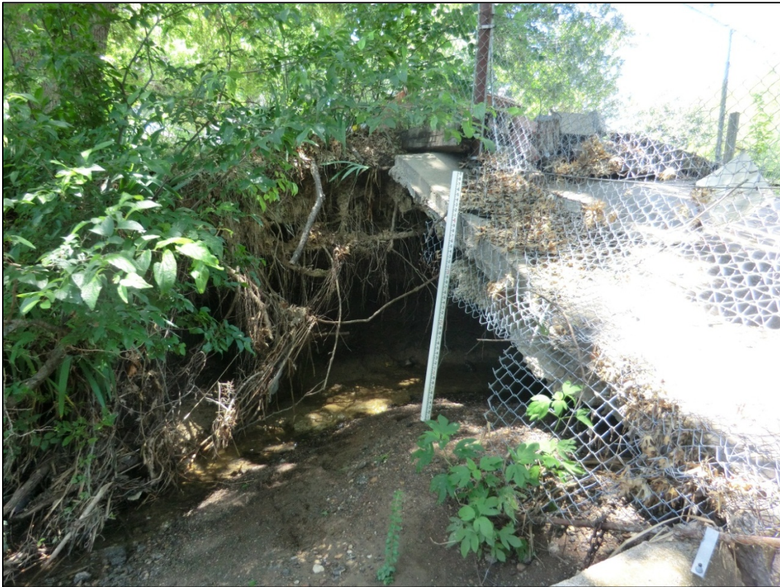
Figure 4.6 Looking upstream at the severely undercut concrete structure near cross section 2272
