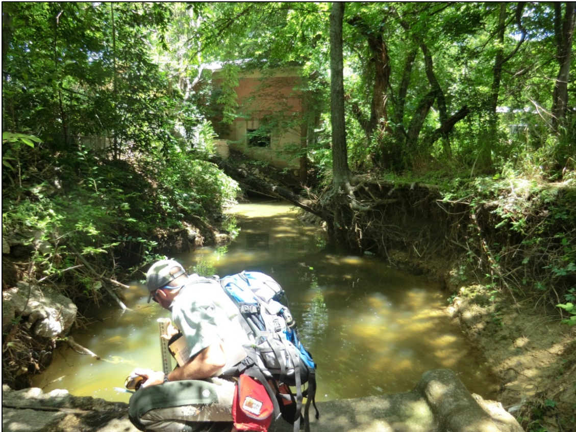
Figure 4.7 Looking downstream at the undercut concrete channel and severe erosion near cross section 2062
