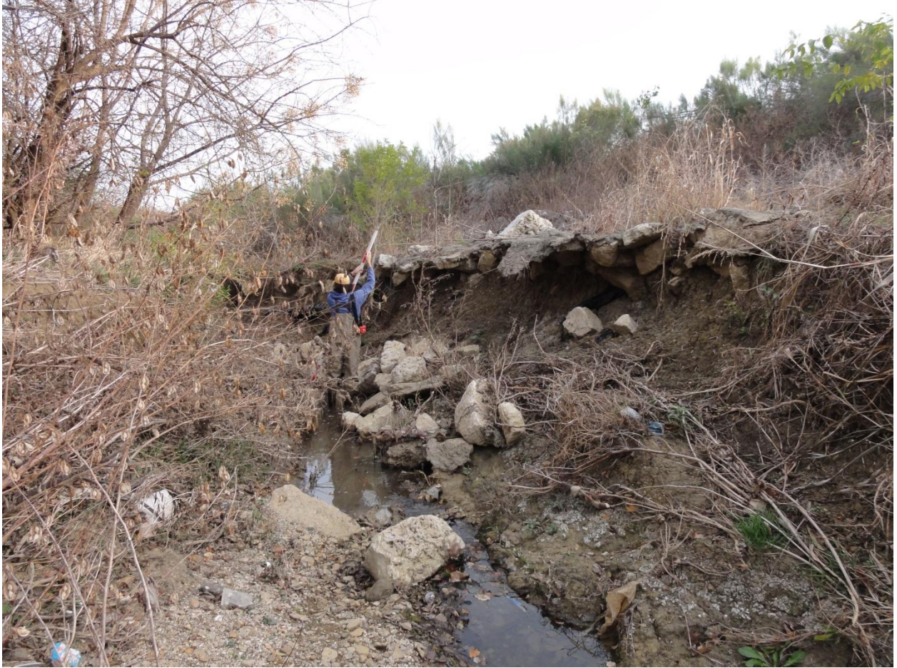
Looking downstream (east) at right bank undercutting and failed protection. Polo Pkwy to the south.
