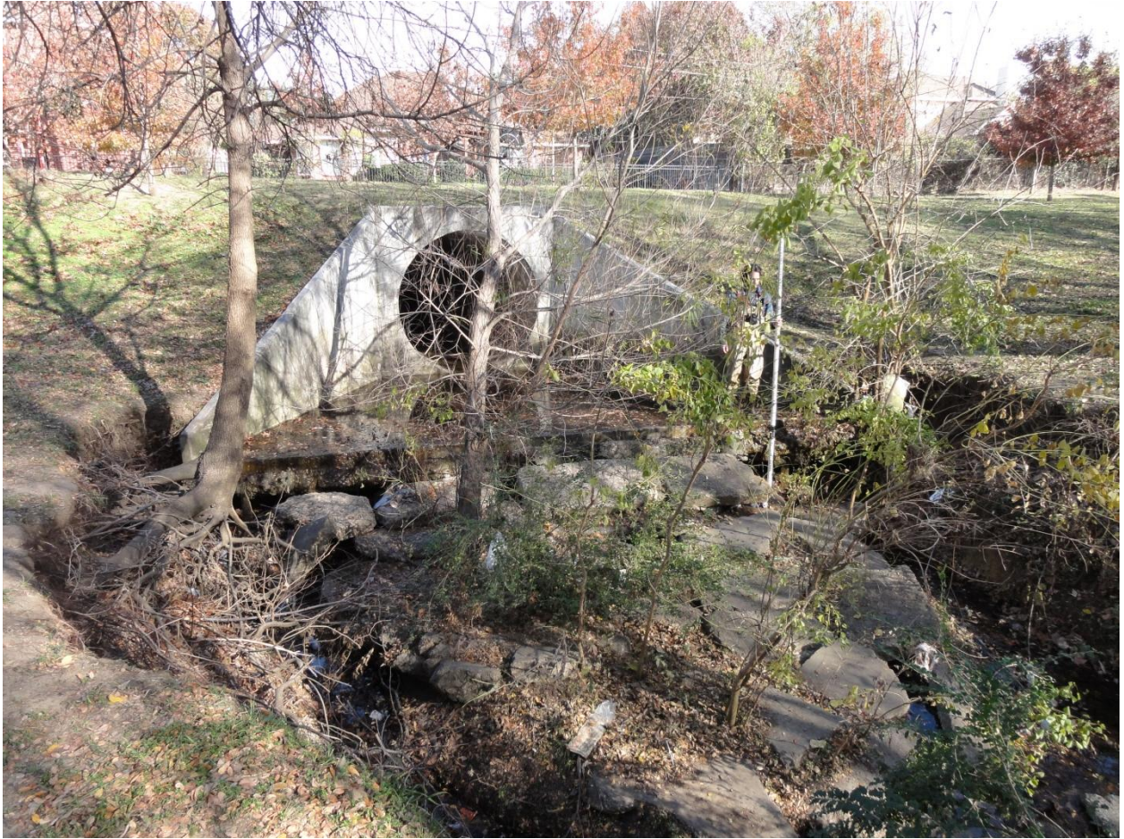
Looking north at 90-inch storm sewer outfall. Headwall/apron scour and failing banks.
