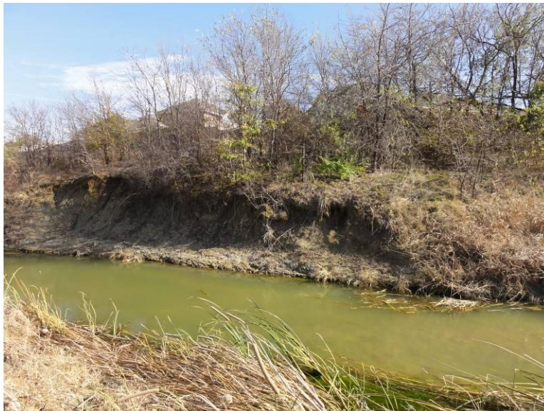
Figure 50. erosion in the channel bank in shale. Increased erosion could lead to upslope problems in terms of potential slumping and earth failure.
