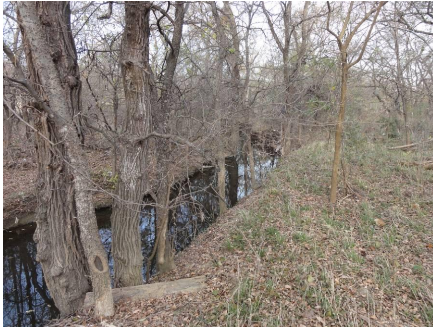
Figure 59. Lower pooled area just upstream of the hardpoint at Bardin. Channel appears stable with little bank or bed scour.
