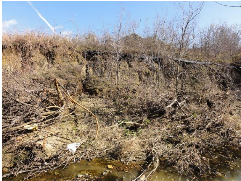
Figure 46. Cutbank erosion with small wedge failures on bank. The top of the house is visible in the background.
