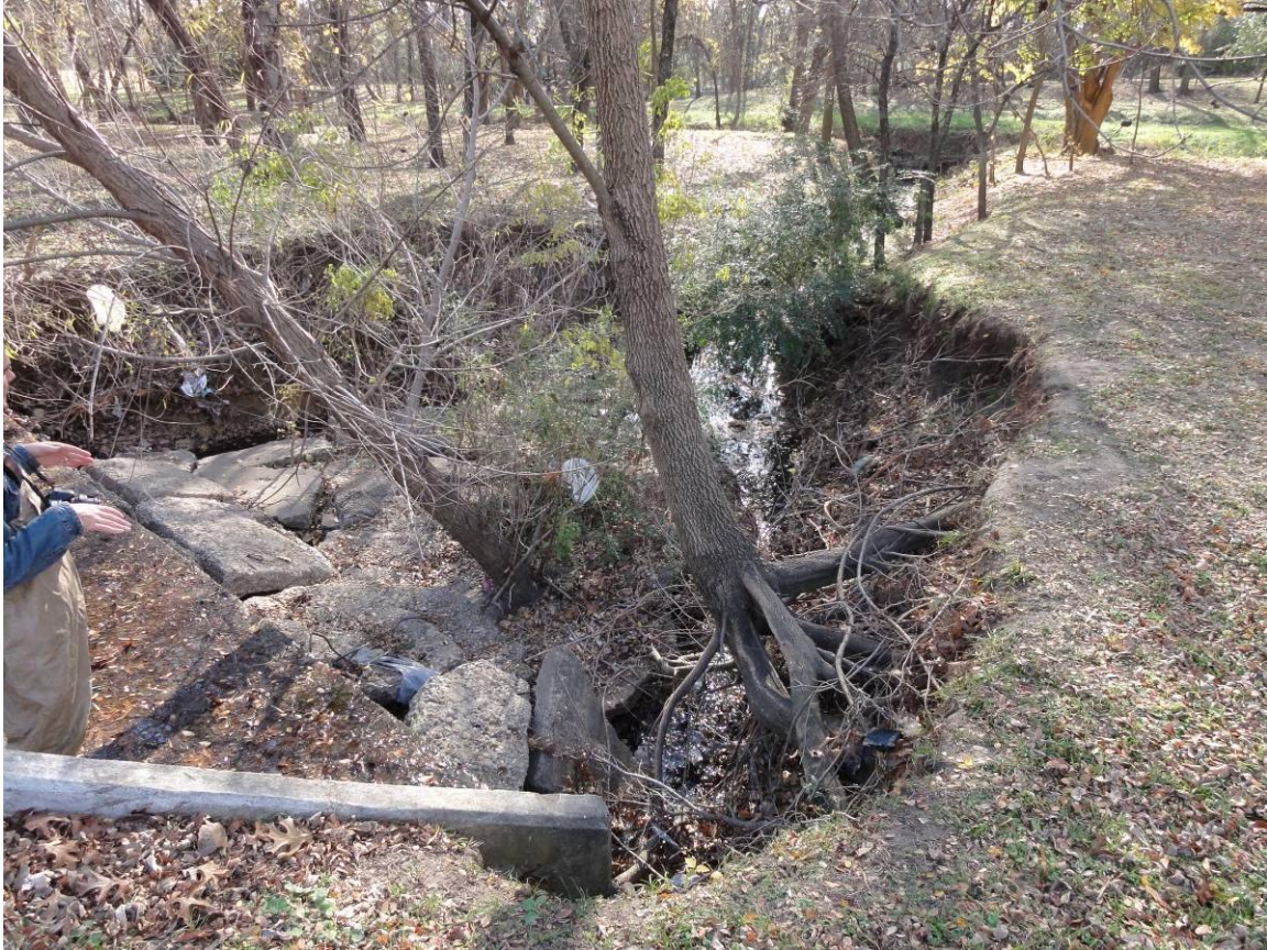
Figure 32. Erosion associated with outfall from large culvert.
