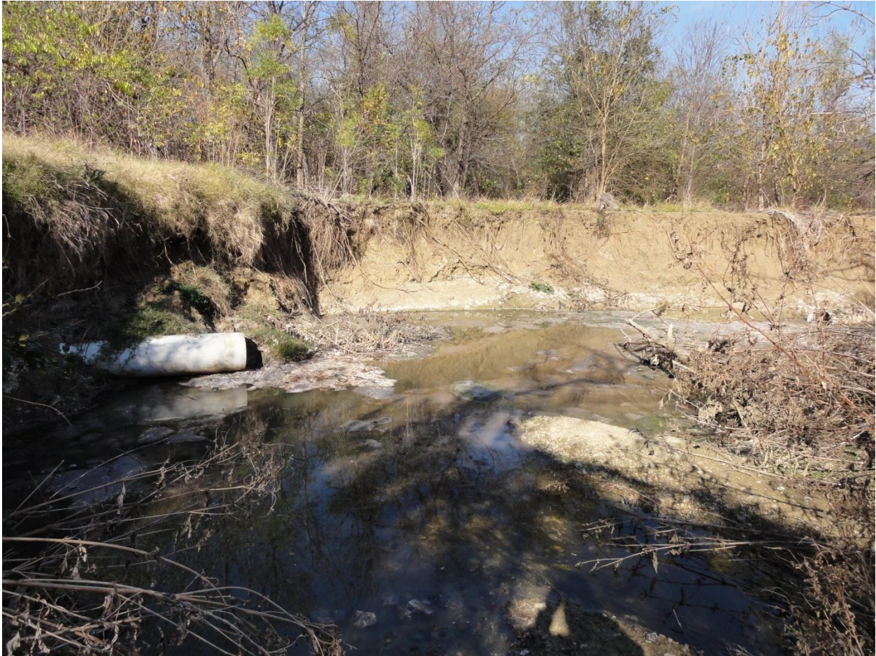
Looking north/downstream at left bank erosion and exposed/broken sanitary sewer line.
