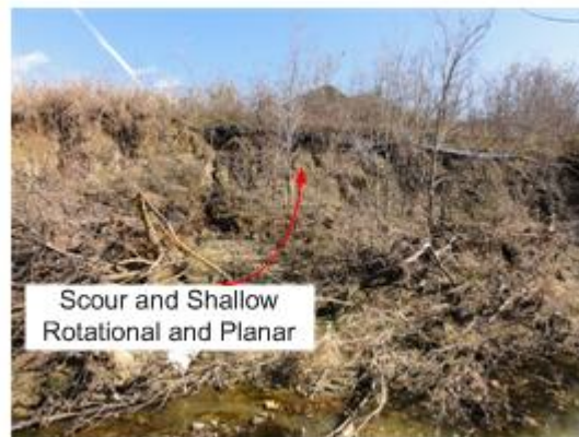
Figure 66. Wedge Failures are common along the outside of meanders or in Type II streams where the channel is incising.
