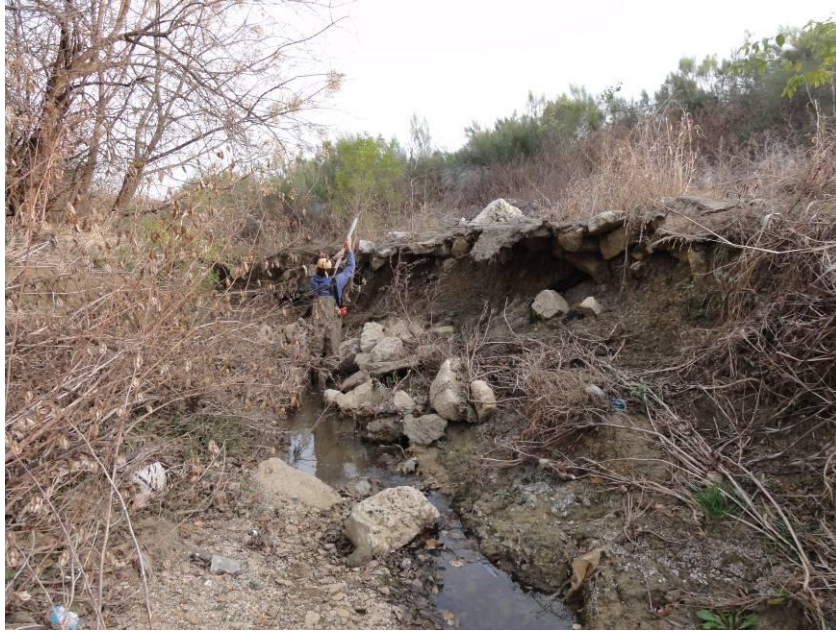
Figure 57. Degrading channel on a meander which is undercutting grouted rip-rap located along Polo Rd.
