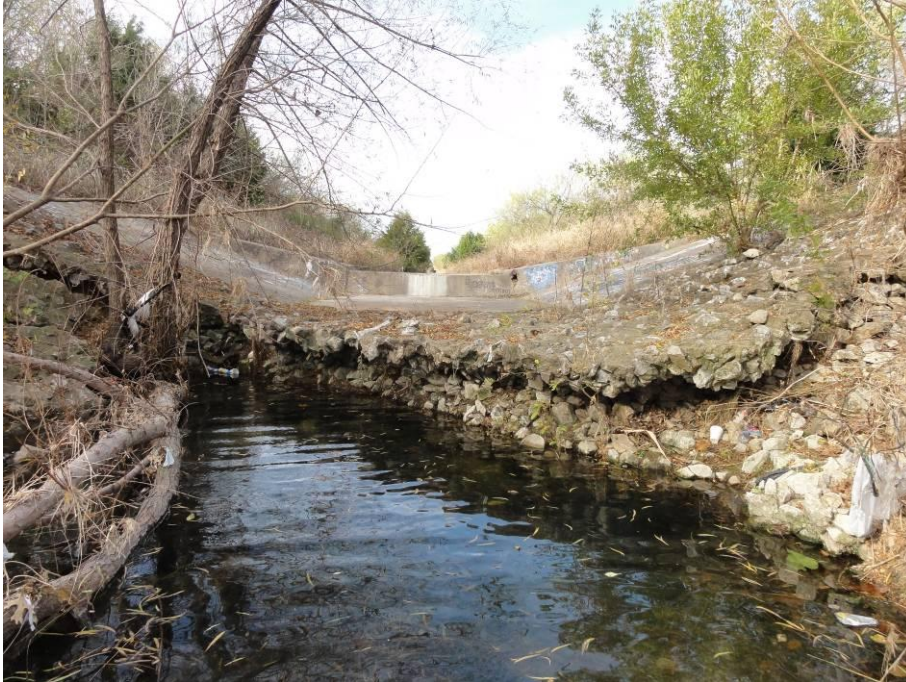
Figure 27. Scour below rip rap at end of channelized section.
