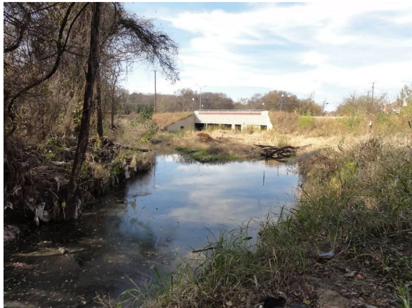
Figure 34. Ponded area and sedimentation (about 1-2feet ) downstream of Carrier Parkway.
