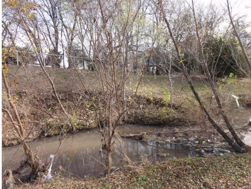
Figure 28. Minor bank scour caused by diversion due to willow growth.
