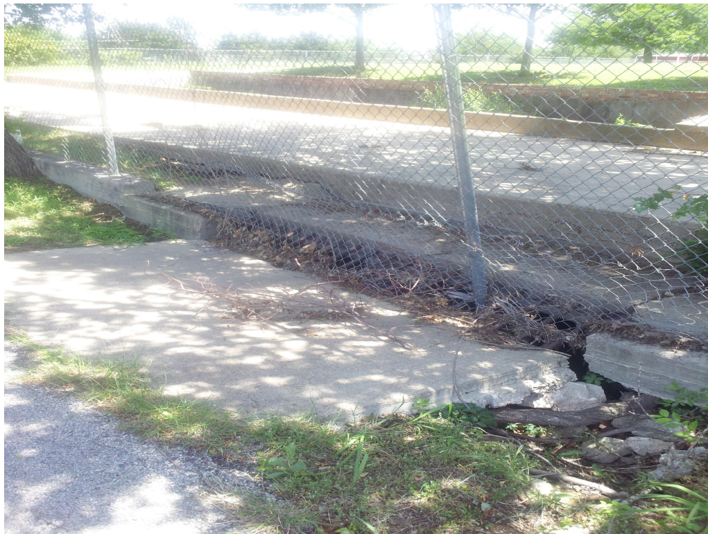
Figure X-5 – Detention Pond Inlet Erosion (facing South-East)
