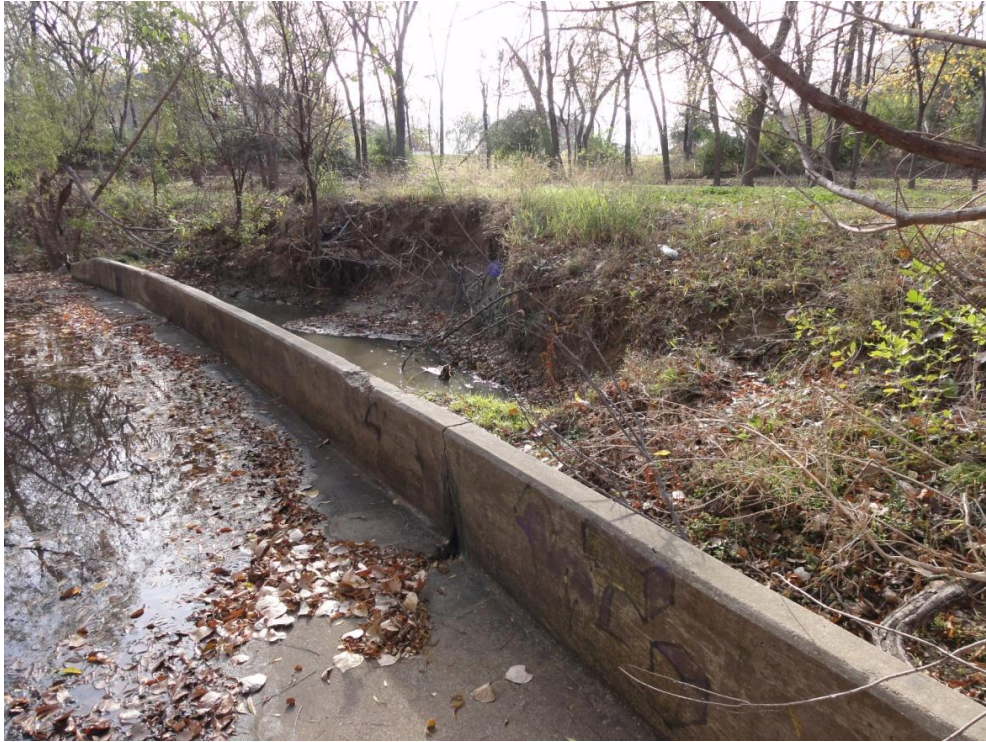
Looking downstream at right bank erosion of concrete flume.
