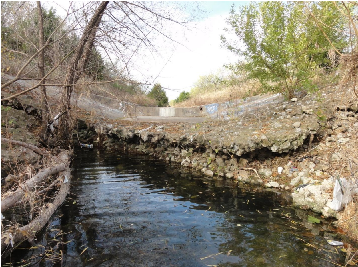
Severe scour; looking upstream at the transition from concrete lined to natural channel.
