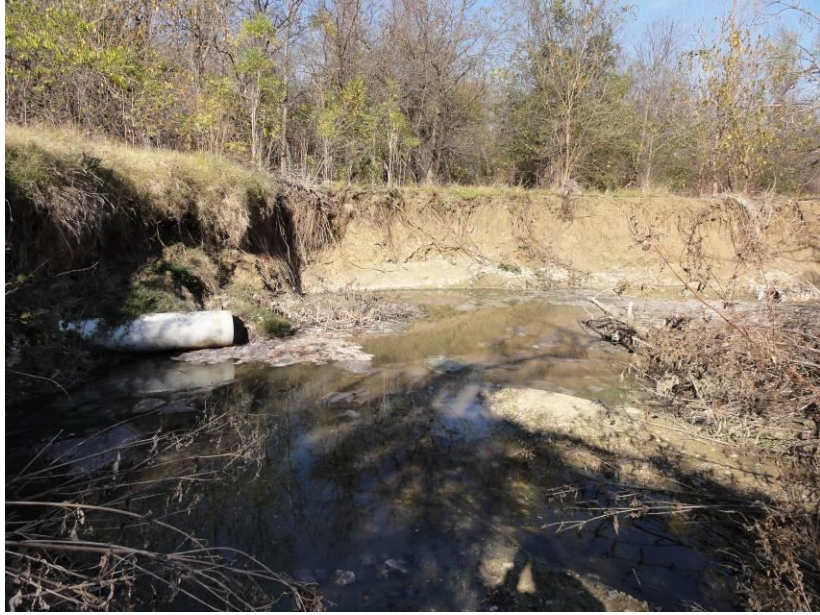
Figure 47. Broken sewer line caused by degradation and widening of the channel.
