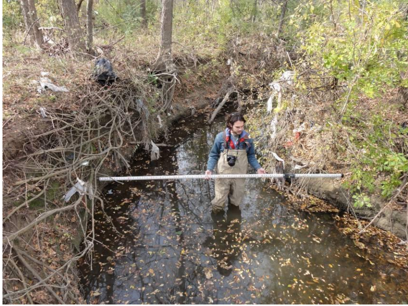
Figure 37. Incising channel and lateral erosion. Bank material silty clay with exposed roots.
