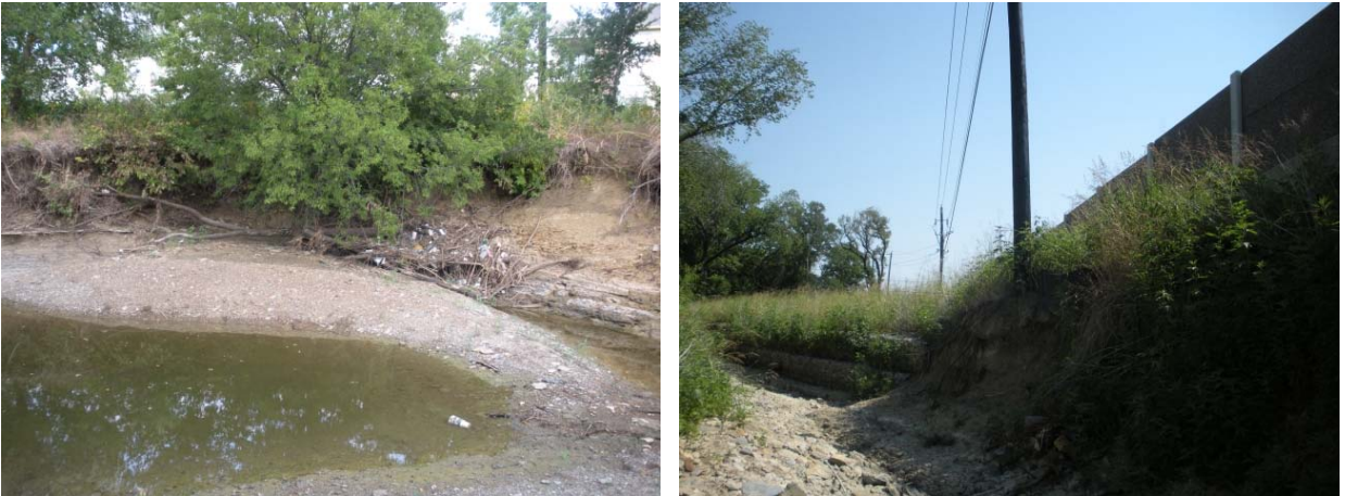
Figure IX-5. Typical Unstable Bank Sections at Station 71+50 (left), and Station 24+77 (right)
