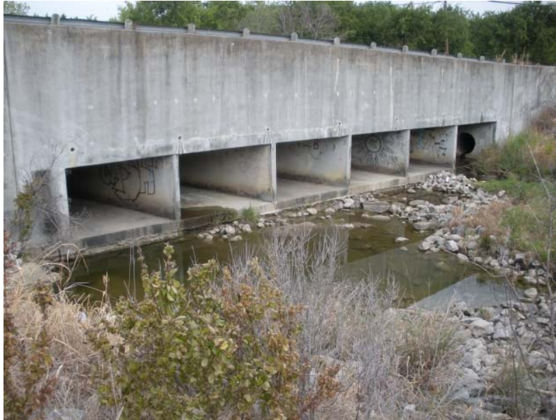
Figure IX-17. View of Scour at the Outfall of the Duncan Perry Road Culvert.
