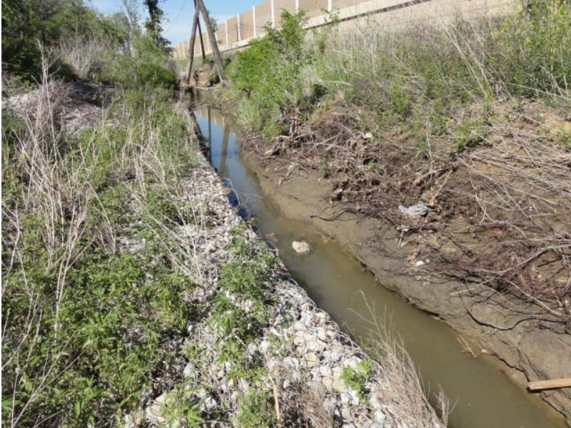
Figure IX-27. Scour Adjacent to Gabion Armoring near Station 26+50
