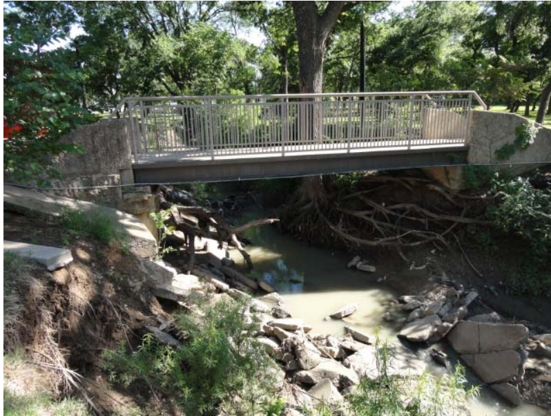
Figure IX-31. Pedestrian Bridge with Substantial Scour (Station 3+50)
