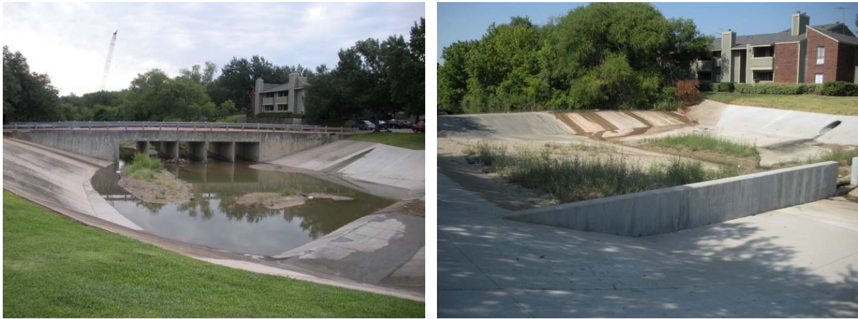
Figure IX-8. View of Sediment in Existing Drop Structures at Station 51+50 (left), and at Station 46+00 (right).
