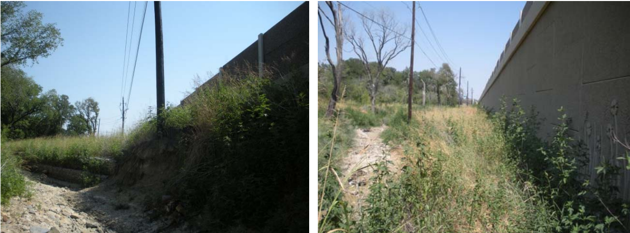
Figure IX-22. Views of Meanders Close to SH-161 at Station 24+80 (left) and Station 30+50 (right).
