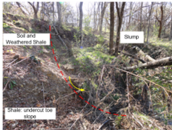
Figure 67. Slump type failure along Arbor Creek (Between Stations 11921 and 12 291). These failures are found where the slopes are typically less than 60 degrees and the stream cuts into an area where the shale is highly weathered or there is soil forming
