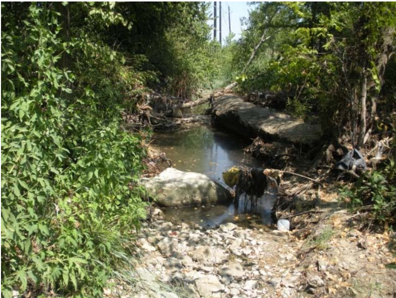
Figure IX-24. Exposed Sanitary Sewer Encasement Near Station 35+50.
