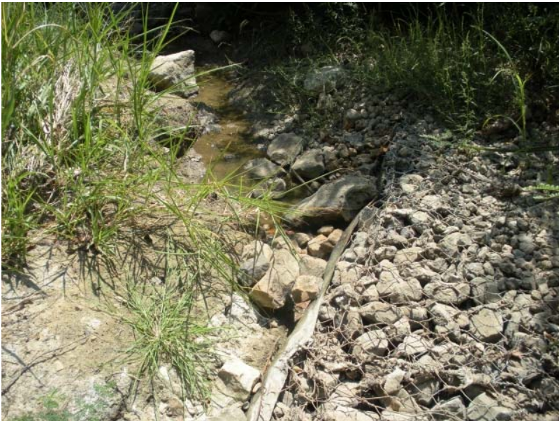
Figure IX-23. Erosion at End of Gabion Mattress Channel Bottom (Station 37+00)
